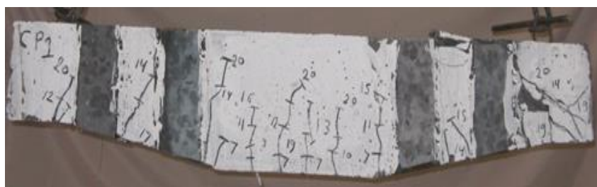
Fig. (33): Crack pattern of beam "CP.1" with thickness of steel plate (2.00 mm)
