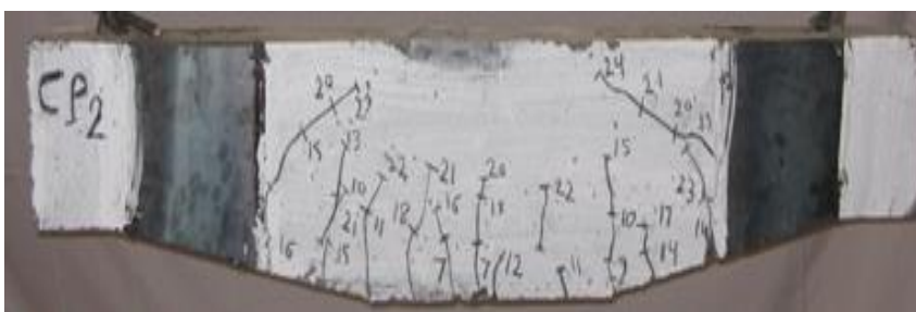
Fig. (34): Crack pattern of beam "CP.2" with thickness of steel plate (2.00 mm)
